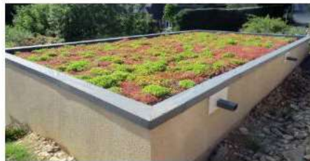
Eco Green Roofs - Sedum blanket
